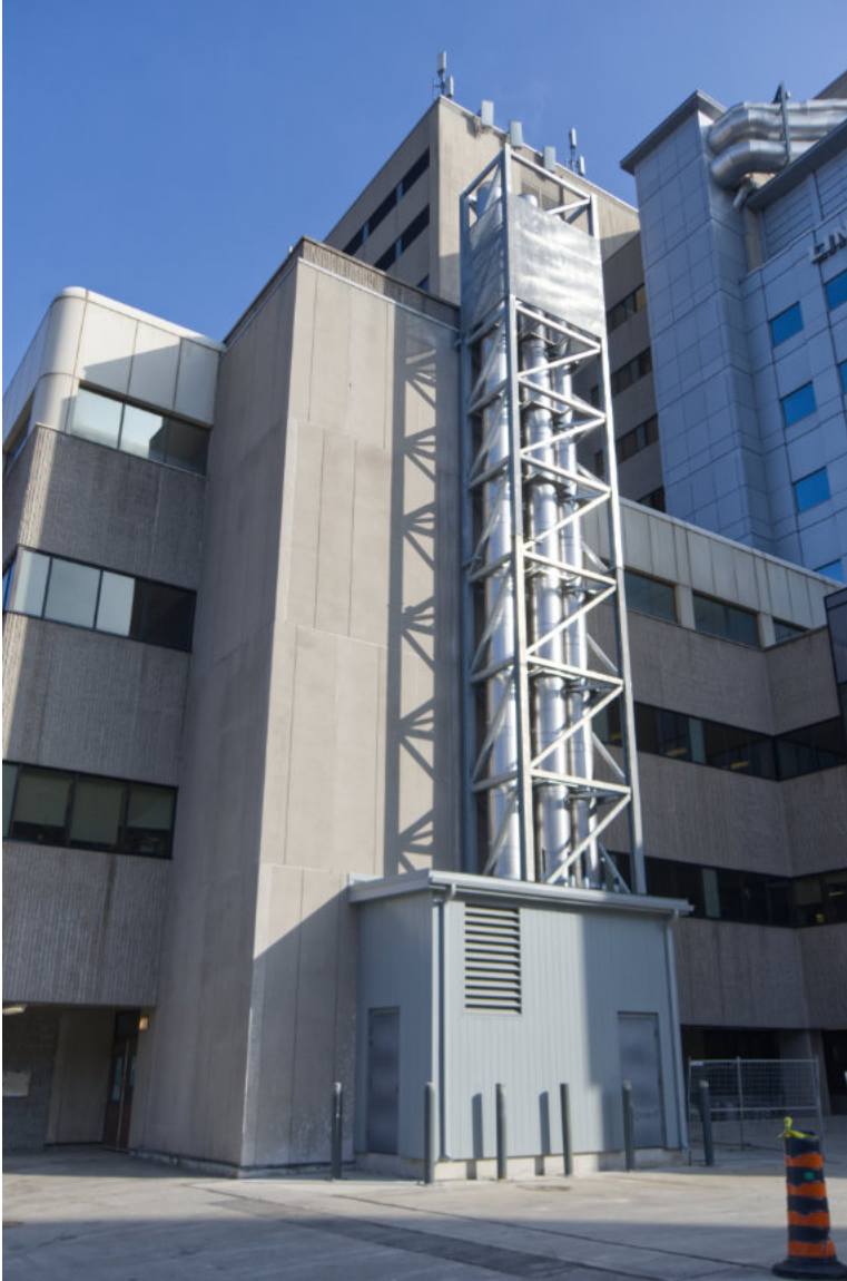
Exhaust stack from the boiler plant
