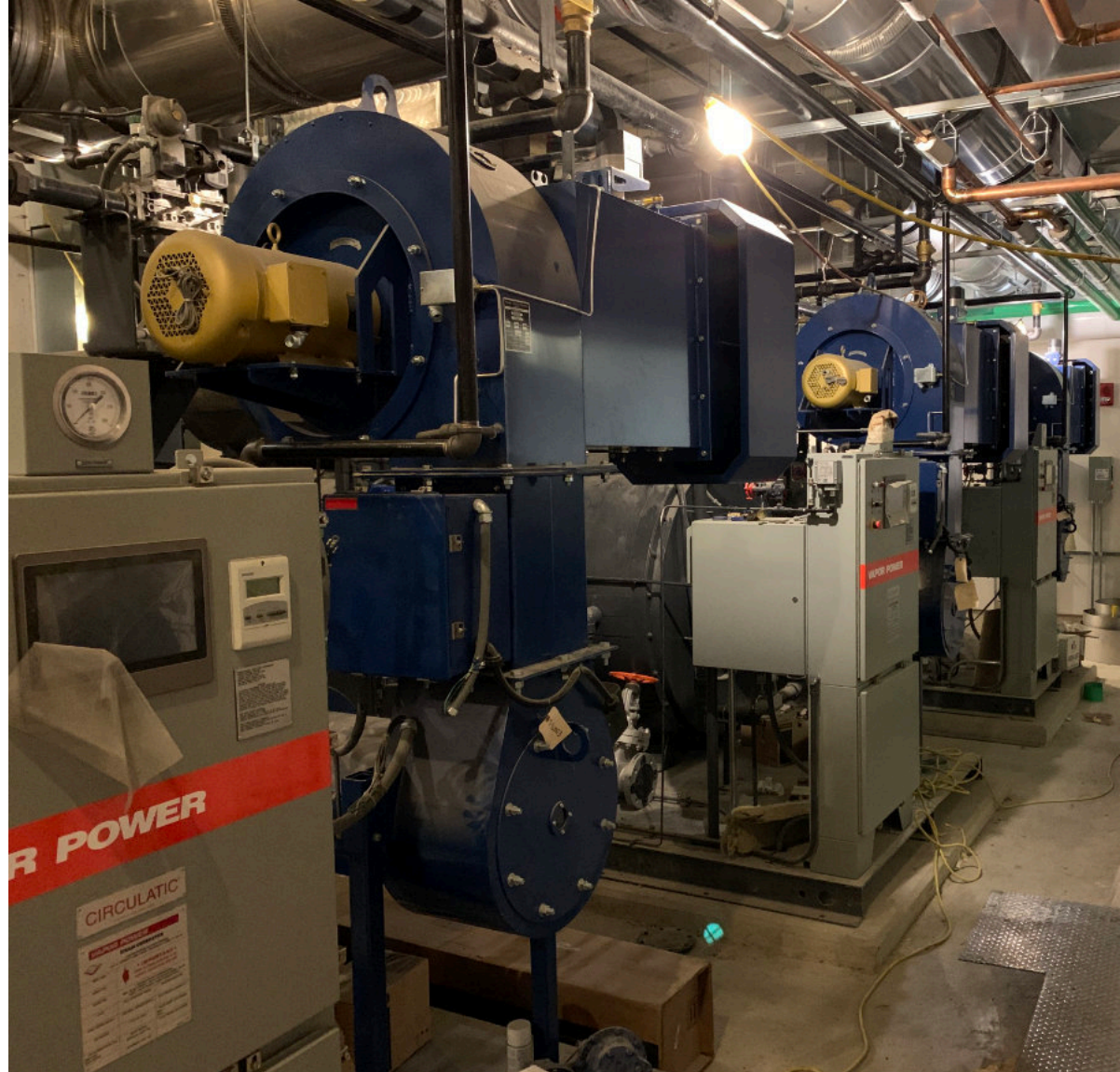
The projects includes three new natural gas fired boilers
