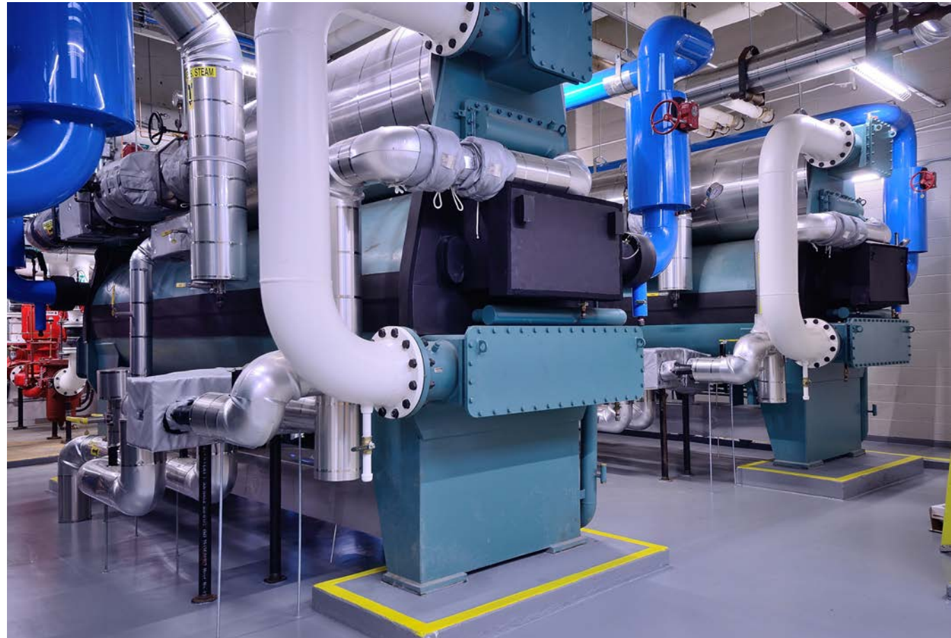
Steam Absorption Chillers at Victoria Hospital are powered by steam produced by our Power Plant, using inexpensive natural gas instead of the local power grid.
